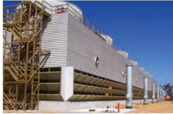
Counterflow Cooling Tower Australia
