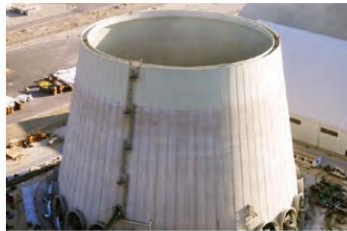
Forced Draft Cooling Tower Dubai
