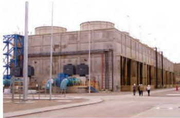
Counterflow Cooling Tower Spain
